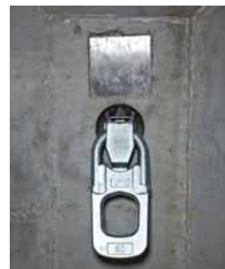
Installed clutch without safety chain
