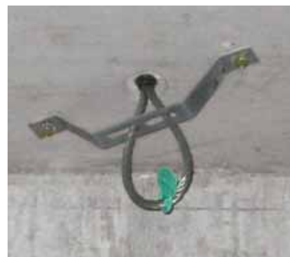
Cable loop installed in a lift head
